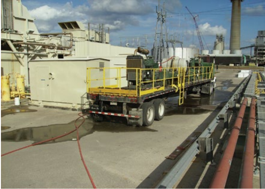
2. Hydrolazing liquid-fuel lines to remove coke is no small task; flatbed holds all the equipment required
